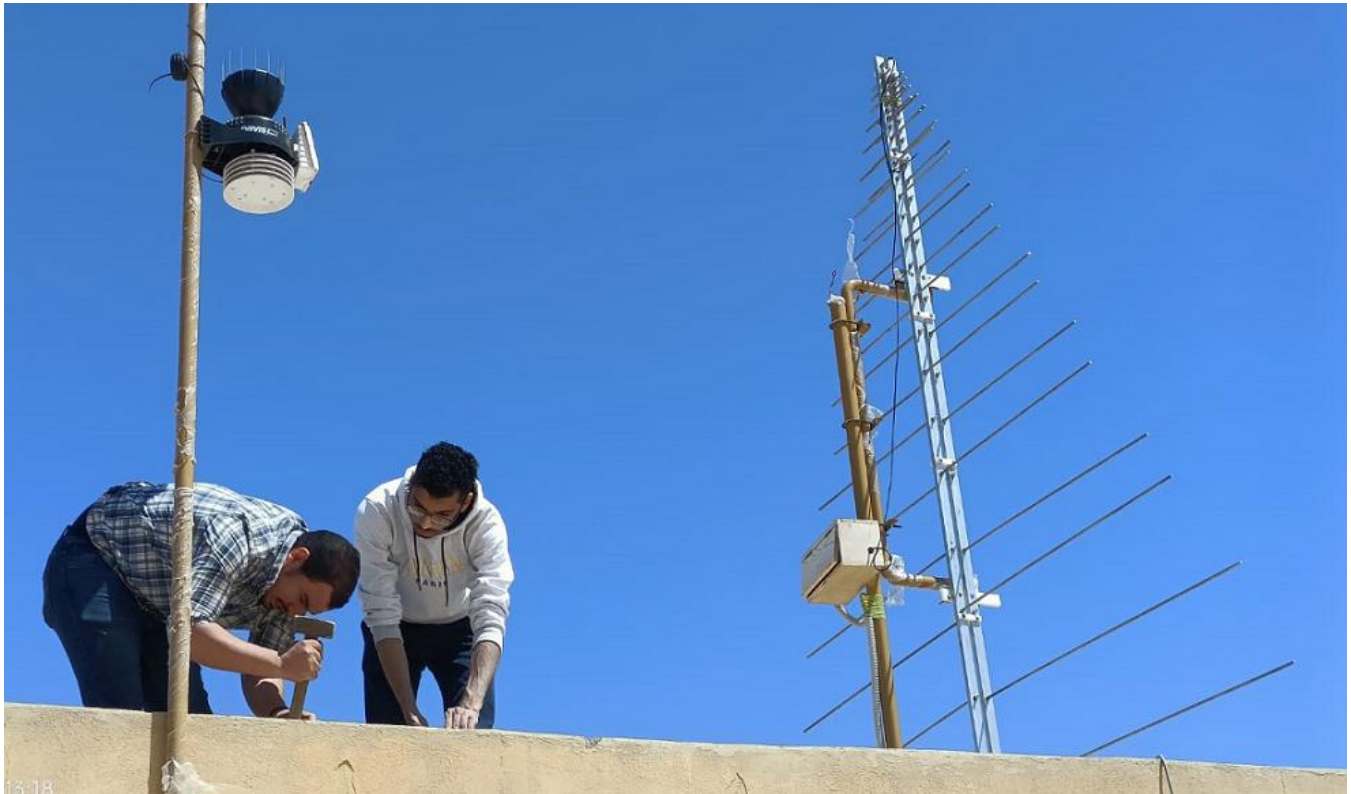
Fig. 2: Installation of LPDA on top of the building. Box contains low noise amplifier
