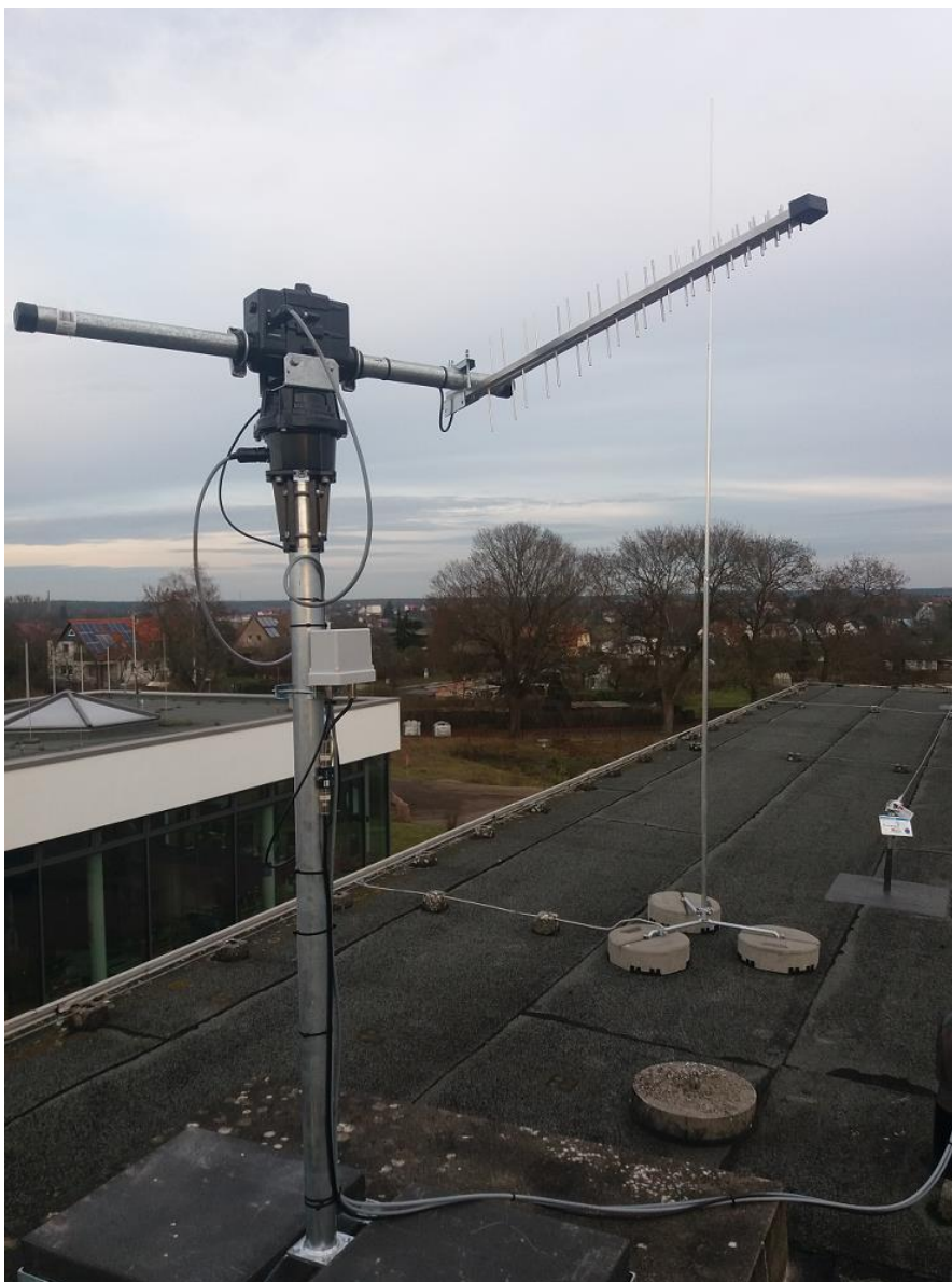
Fig. 1: New antenna installation at DLR in Neustrelitz, Germany. LPDA in vertical polarization for L-band including tracking system.
