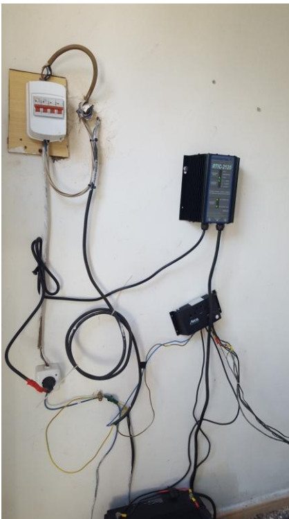
Fig. 2: 3-phase circuit breaker, PV-controller and power supply for seismometer.
