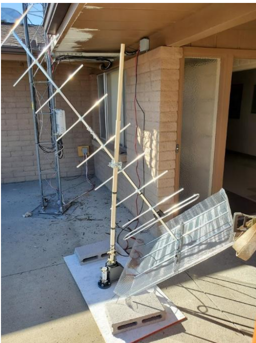
Figure 1: Antenna System and mount
