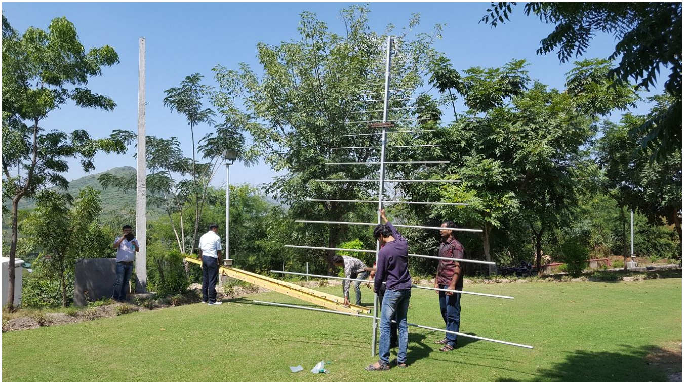
Fig. 1: Preparation of LPDA for mounting on a concrete pole at PRL in Udaipur, India.
