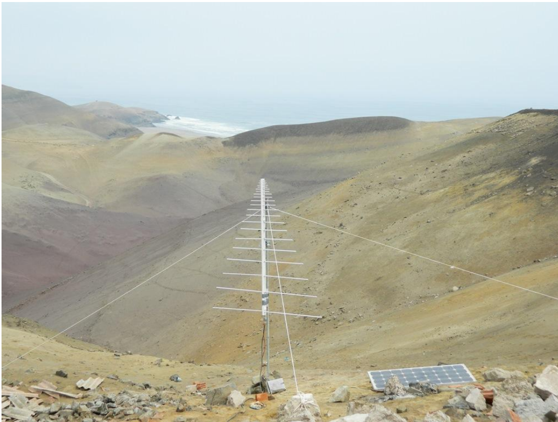
Fig. 2: LPDA in a very rural area in Punta Lobos, Peru 76,79889 W and 12,51 S. Photo voltaic panels to supply electrical power.
