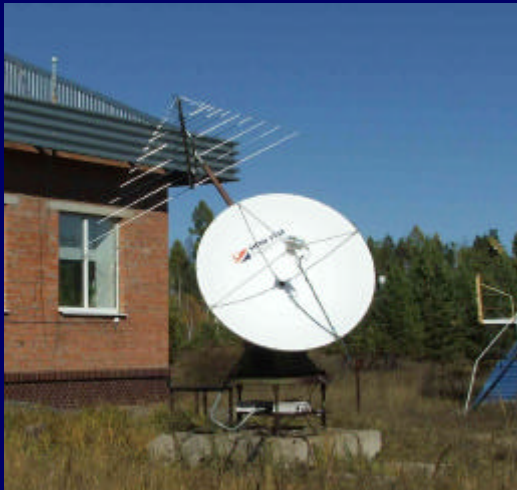
Antenna attached to dish
