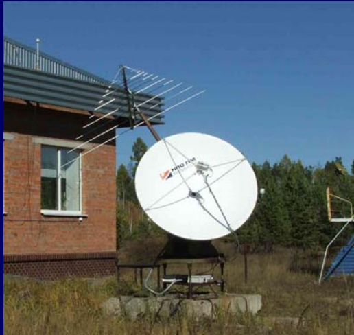
Antenna attached to dish
