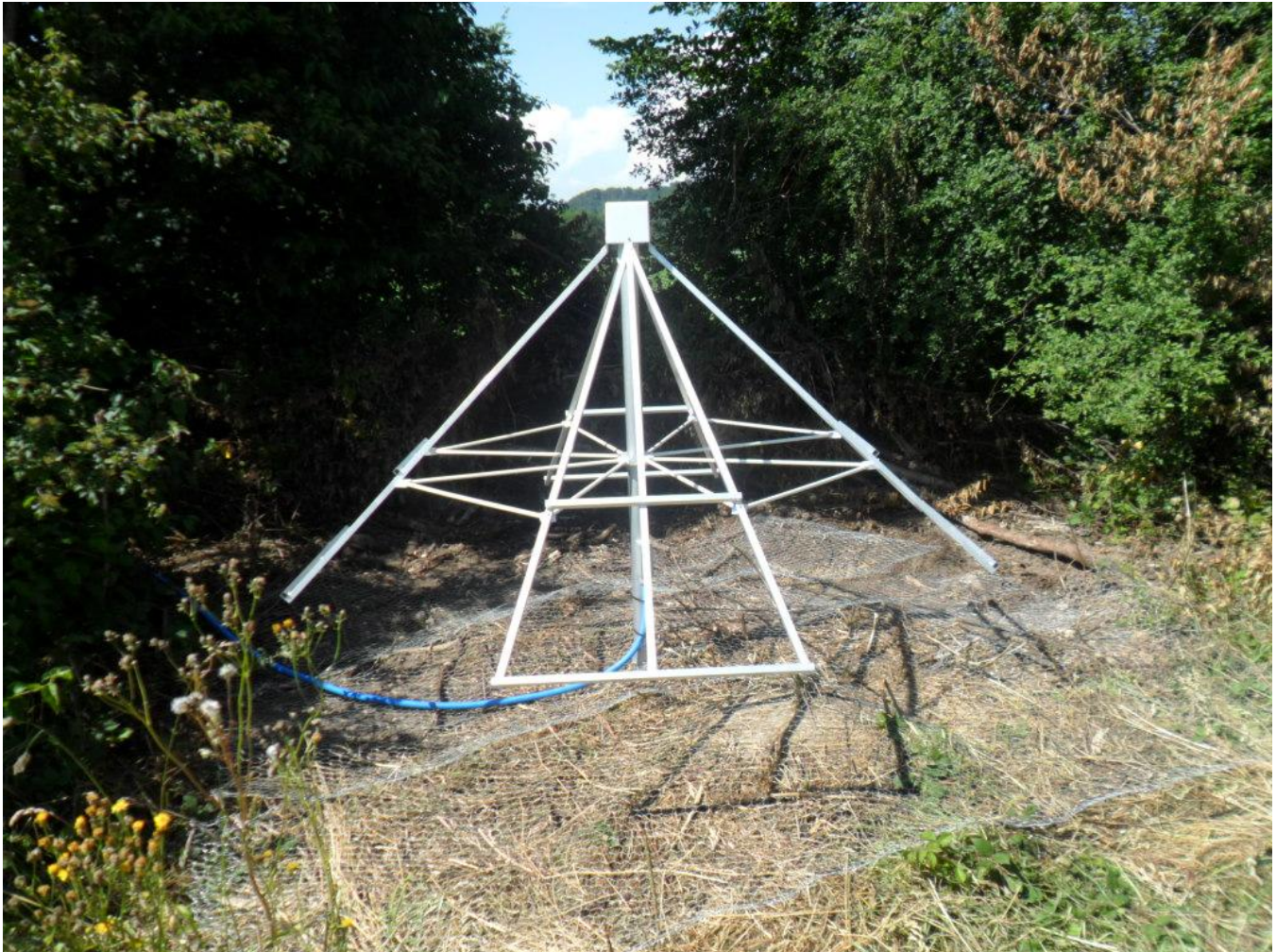
Figure 1 ~ An LWA antenna installed at the observatory site in Bleien, Switzerland. Chicken wire mesh on the ground functions as ground reflector to improve antenna gain and its beam pattern. The blue plastic tube contains two coaxial cables (one per linear polarization) going to the observatory. I am not allowed to cut the nearby bushes because the antenna site is in the center of a protected natural zone for birds.
