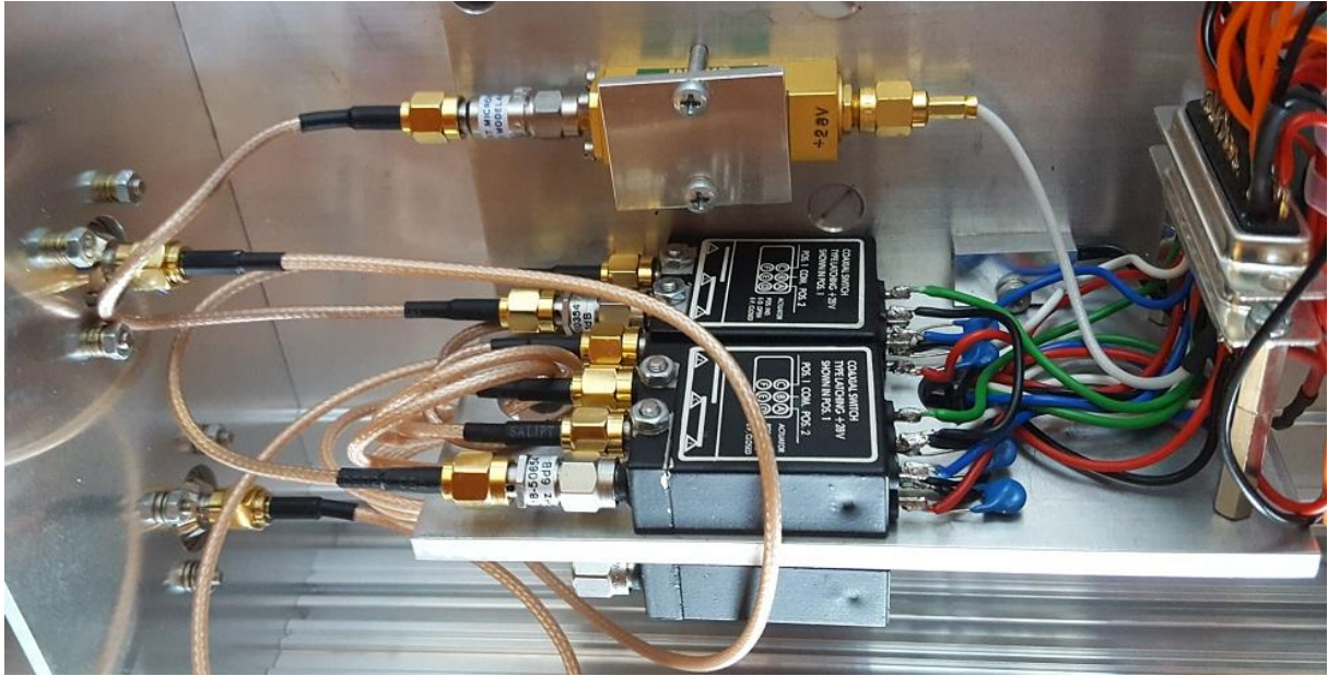
Fig. 3: One half of calibration hardware with noise source, attenuators and microwave relays.
